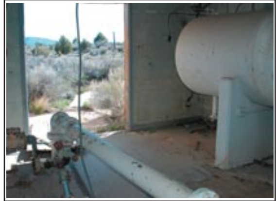
Figure 2.38 Building #11, Water Storage Tank
