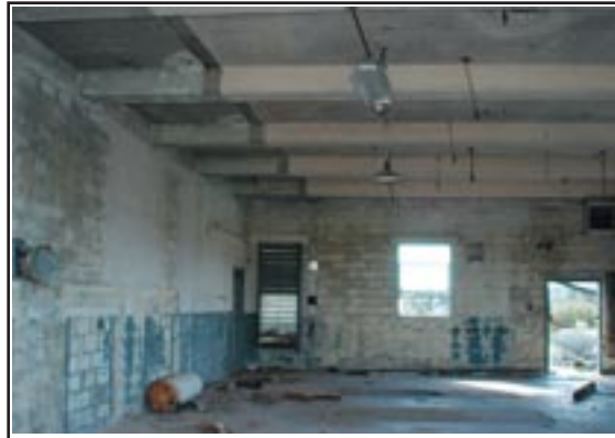
Figure 2.18 Interior, Building #2, Electric Primary Power
