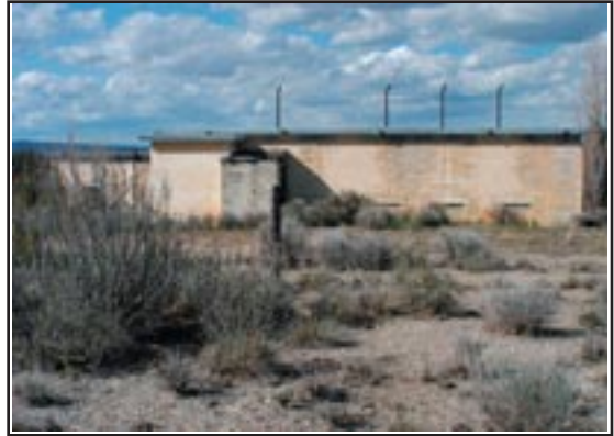
Figure 2.17 South Facade, Building #2, Electric Primary Power
