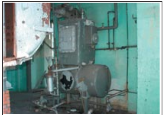
Figure 2.22 Portable Boiler, Building #4, Heating Plant
