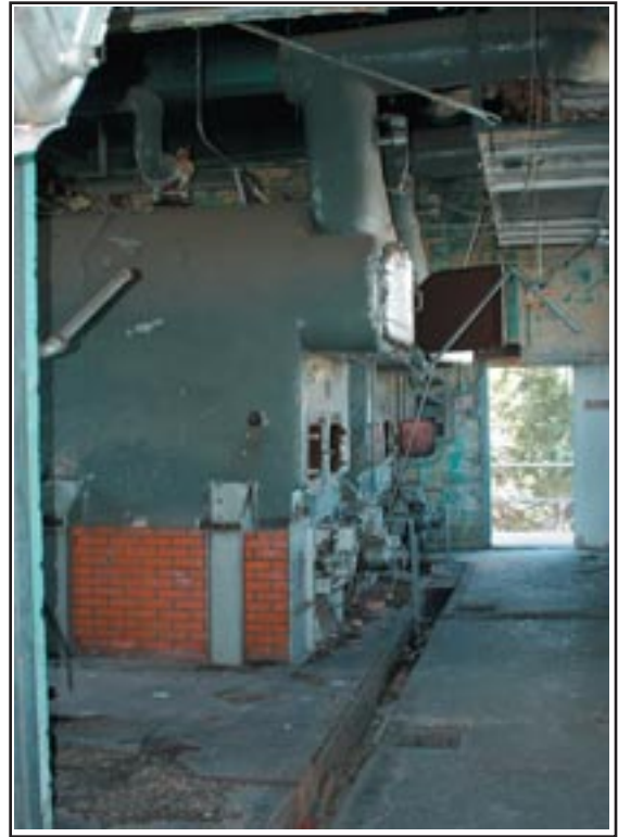
Figure 2.21 Boilers, Building #4, Heating Plant
