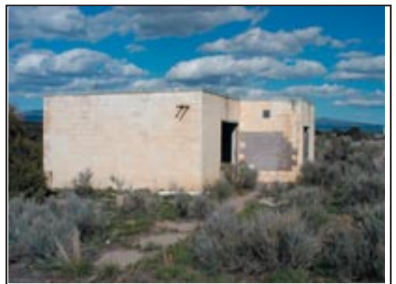
Figure 2.37 Building #11, Water Supply Treatment
