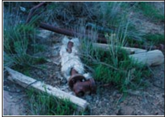
Figure 2.11 Pipe with suspected asbestos insulation
