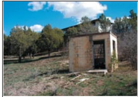
Figure 2.36 Building #10, Water Pump Station
